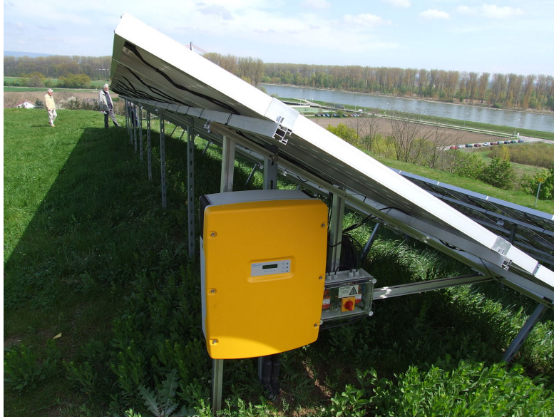
Figure 7: Inverter Connected to Solar Panels
